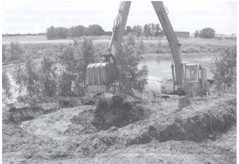
An earthmover removes material from one of the silt traps in the Potowolonga catchment.
